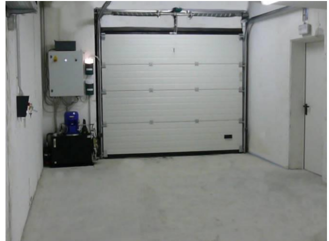
Sectional door application in the basement
