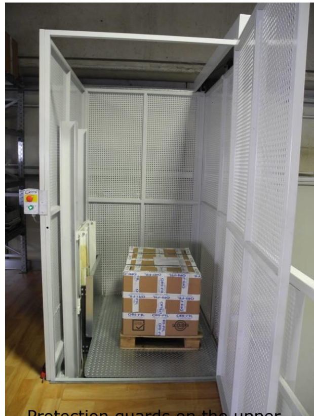
Protection guards on the upper floor with door gate and safety electric lock
