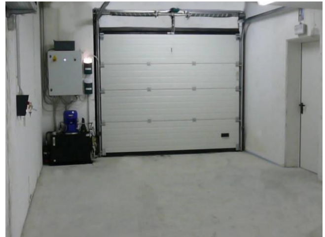
Sectional door on underground level
